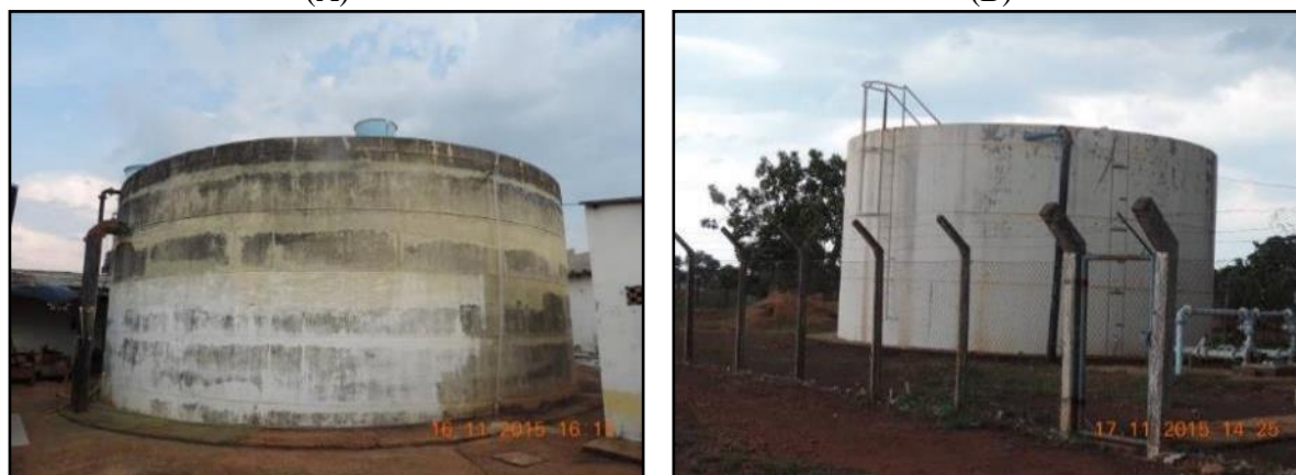
Figura 11. Reservatórios: RAP-01 (A), RAP-02 (B), REL-01 (C) (A) (B)
